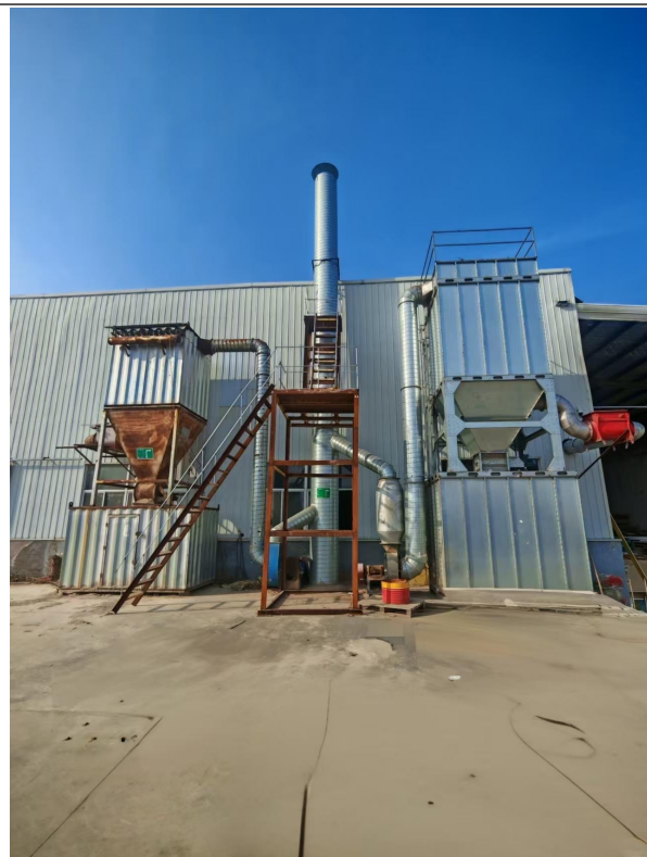
脉冲袋式除尘器+3#排气筒
